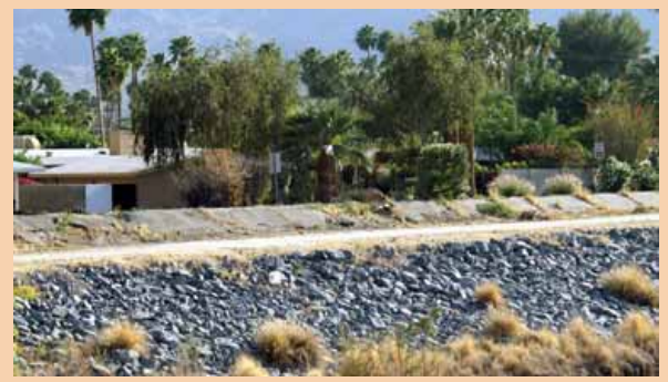
Failing berm and dead oleander
